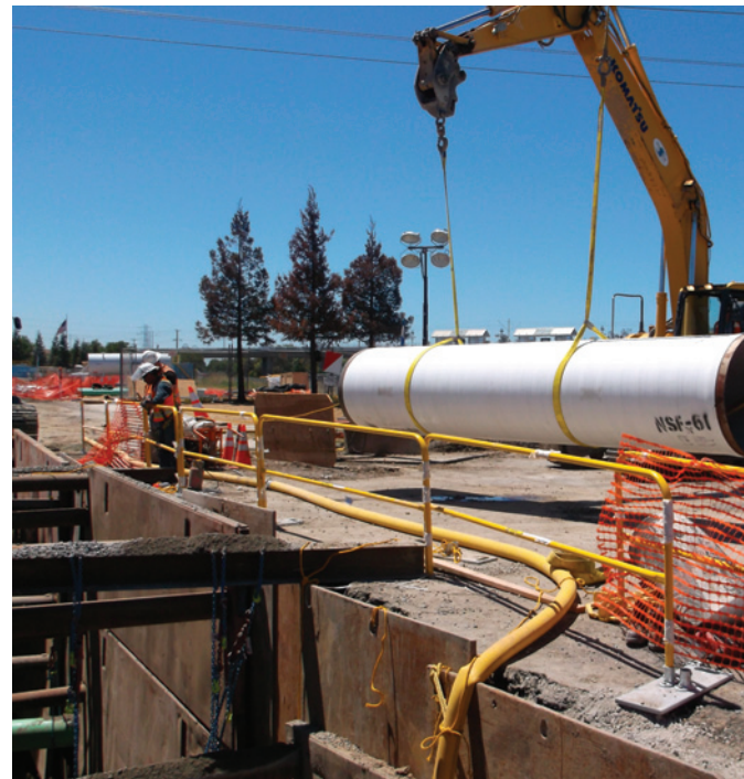
VTA AND the project team relocating a large diameter water pipeline owned by the Santa Clara Valley Water District for the BART Silicon Valley Extension. Project Fact sheet at MassTransitmag.com/12296322
